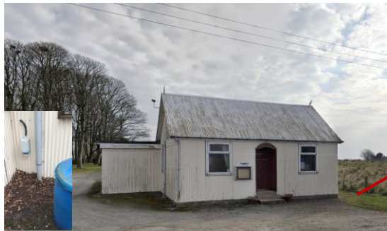
Whiterashes Hall Changeover Switch Installed
