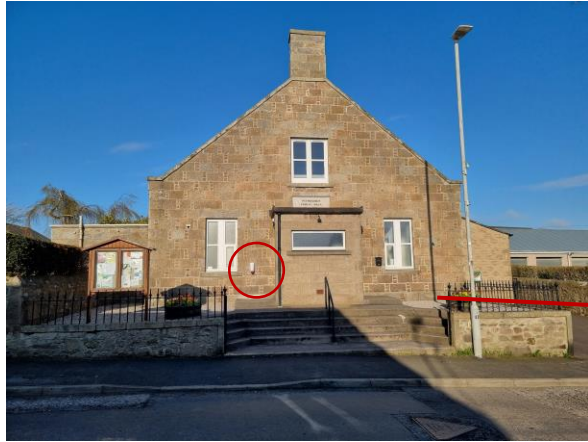
Pitmedden Hall Changeover Switch Installed
